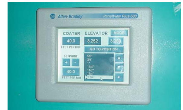
Automatic Elevator Control Panel
