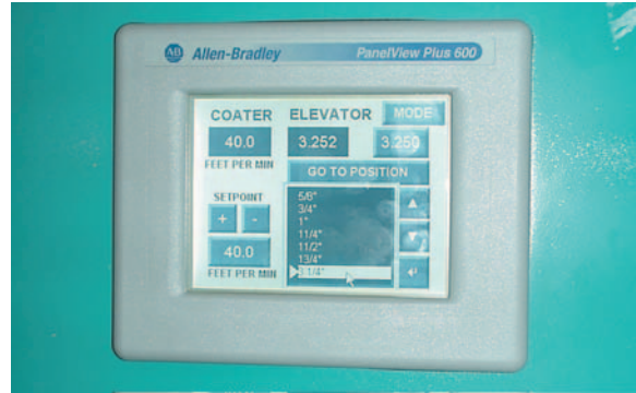
Automatic Elevator Control Panel
